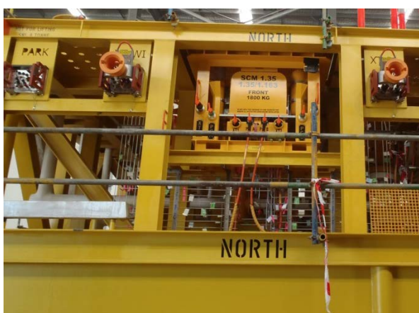
Fig. 1: Subsea Manifold, Retrievable Subsea Control Module (SCM) and Sacrificial Anodes
